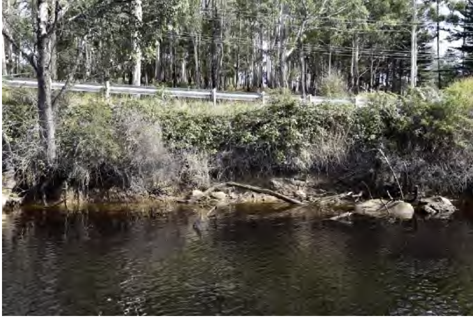
Plate 30 Fallen trees and erosion adjacent the road
